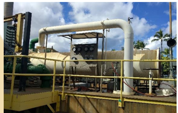
Figure 2: Shell and Tube Heat Exchanger at Kahe (HECO)
