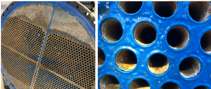
Figure 4: Left: HeatX-treated heat exchanger after 26 months in service. Right: Tube sheet after a simple pressure wash.
